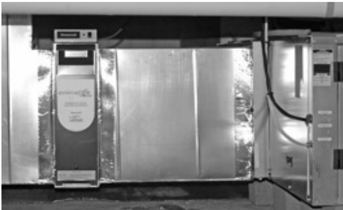
Geothermal unit in conditioned crawl space.
